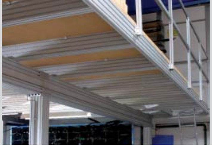
Individual platform as warehouse mezzanine
